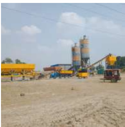
Wet Mix Macadam Plant / CTSB Plant
